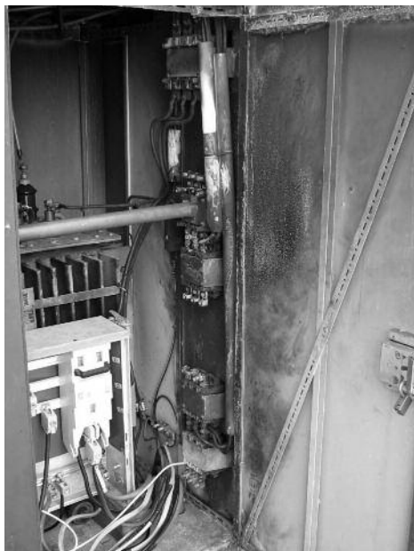
Brandskaded transformerstation i Ærøskøbing.
